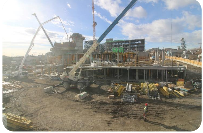
Mobile cranes on site. Formwork for columns main to second floor and second floor slab being installed.
