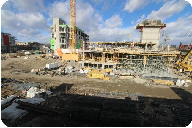
East tower concrete is complete and exterior framing in progress. Elevator shaft walls almost complete.
